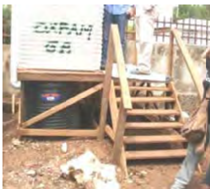
Figure 29. Single cubicle tanks
