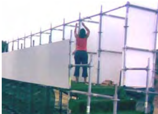
Figure 10. Toilet framework of steel scaffold poles
