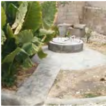
Figure 38. Biogas plant in Port au Prince
