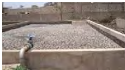
Figure 54. Sludge drying bed
