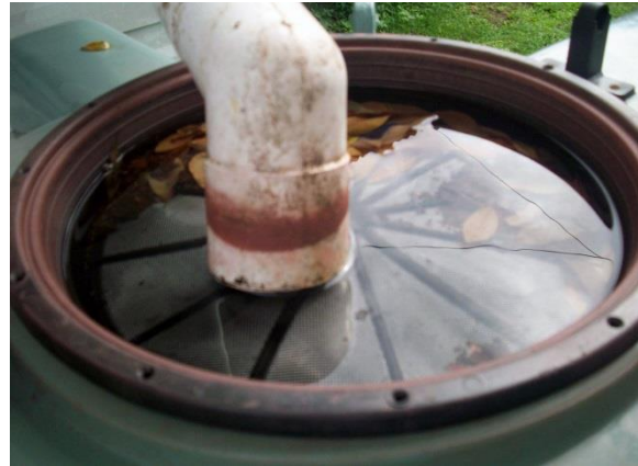
Image 5.1: Water overflowing through inlet screen due to absent outlet
