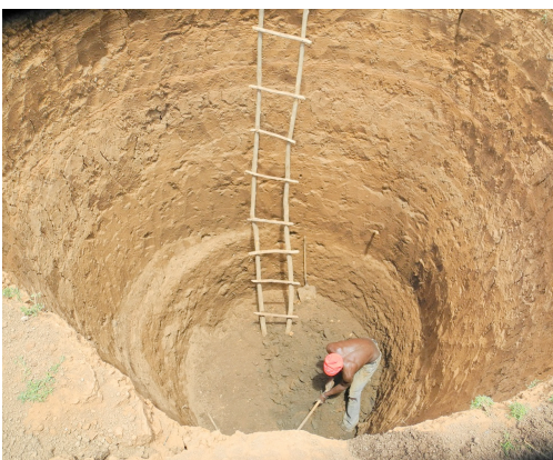
Photograph 5. No water at 3M deep WELL prior to desilting
