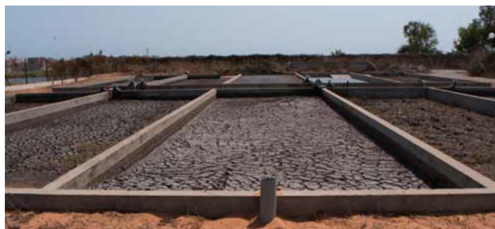
Photograph 2. Drying beds at Niayes faecal sludge treatment plant, Dakar, Senegal
