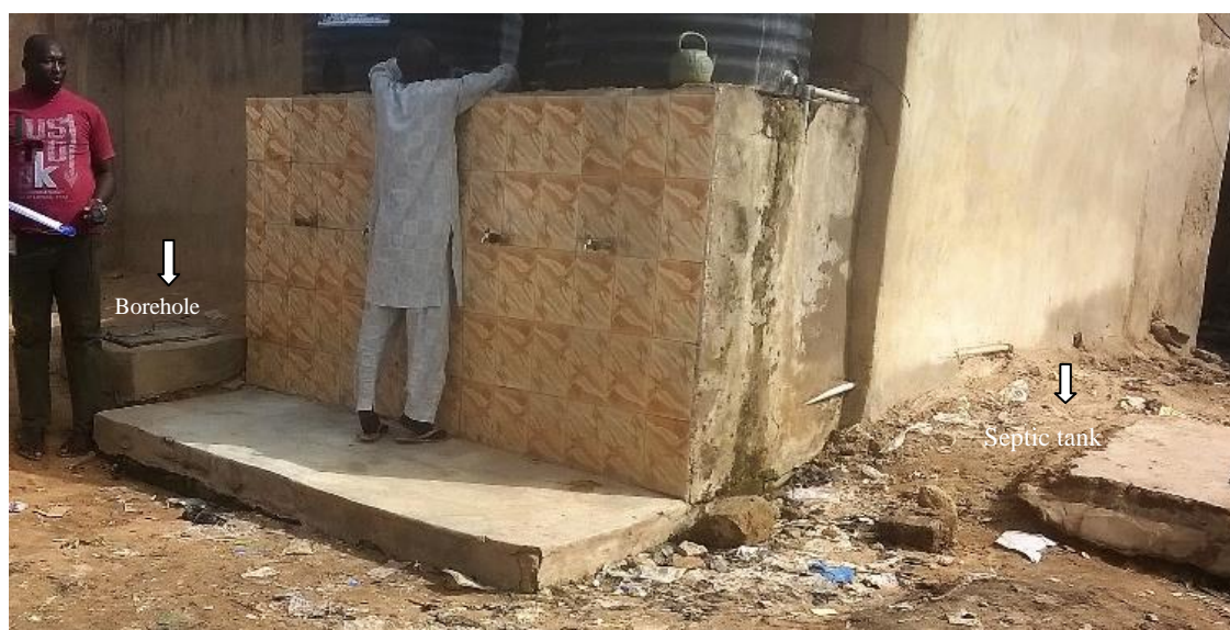
Photograph 1. Public water supply with borehole and septic tank
