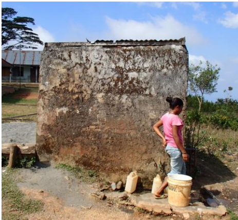
Photograph 1. Water tank without a water level indicator
