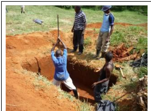
Photograph 1. A recharge hole is made with a Soil punch. This hole passes the compact clay layer and in this case is 5 meters deep
