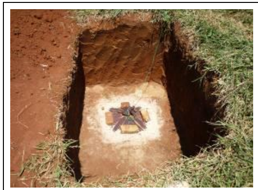
Photograph 2. The hole is filled with gravel and covered by a sand filter that is then covered with a cloth filter. A rope is attached to the cloth filter to pull it up for cleaning
