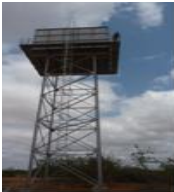
Photograph 2. Elevated tank, Dadaab
