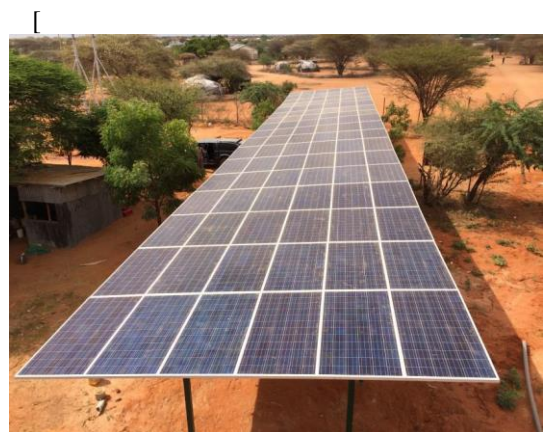
Photograph 2. Solar panels array
