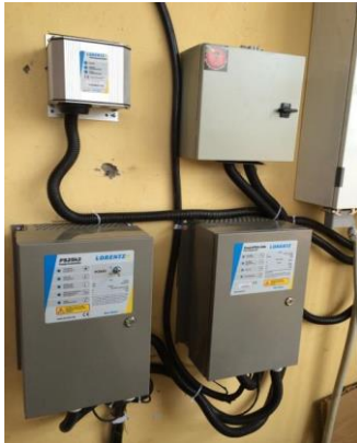
Photograph 1. Submersible pump controller, power unit and communicator
