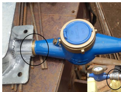
Photograph 3. 1" multi jet water meter directly screwed onto a U2 water tank (connection emphasized by circled area). The inset shows what the connection was like before this modification.
