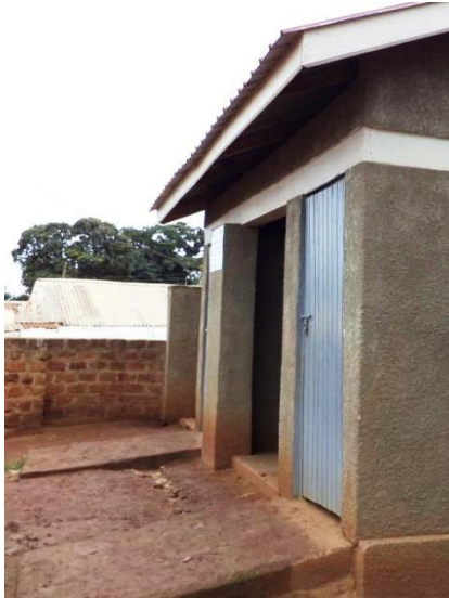
Photo 1. Ramps with gradient 1:12. Note lack of platform at top of ramp and high door bolt. This would be inaccessible for a wheelchair user. (Kasumba 2012)
