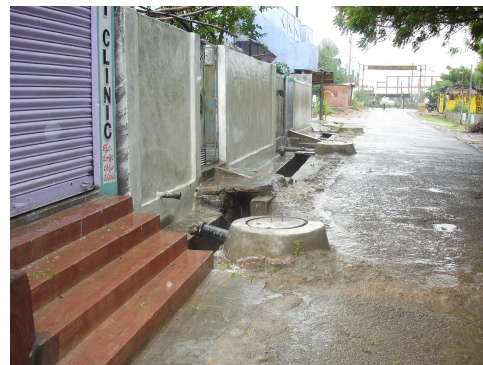
Photograph 2. A shallow chamber for house connection
