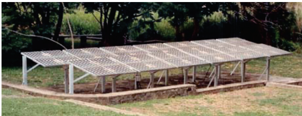
Figure 2. Solar array used in testing
