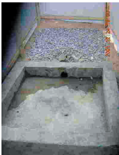
Photograph 3. Washing slab for menstrual cloths inside a screened block
