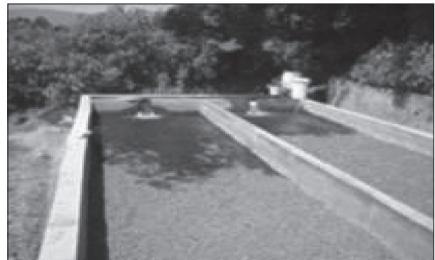
Photograph 1. Short circuiting of DRFs at the inlet
