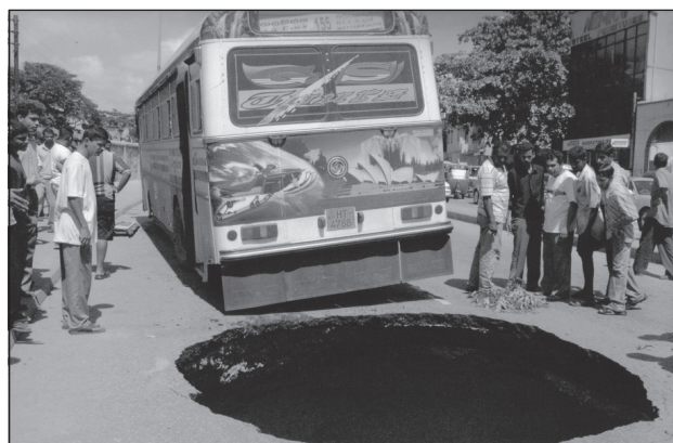
Figure 1. Road collapse in T. B. Jayah Mw in Colombo, September 2005
