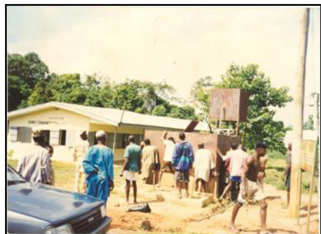
Picture 1. The type "A" water supply scheme located by the side of the community hall
