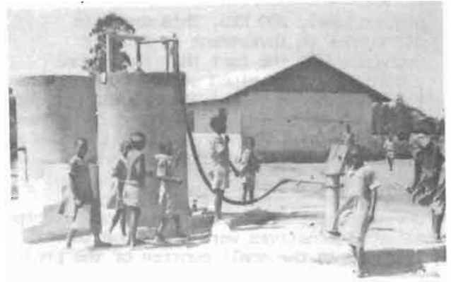
Iron removal at Lusumu Primary School. The handpump is locally made.
