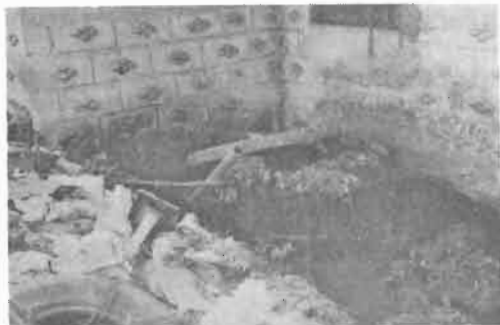
Figure 1. Raw sewage spilling from a manhole forms a rivulet running to an open drain in the Sonnewein sector of Monrovia. The manhole is on a sewer permanently blocked by sand and grit.
