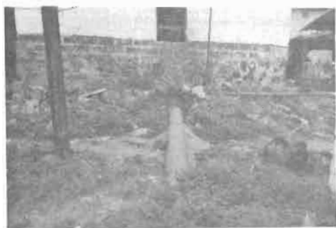
Figure 2. A house has been constructed directly on top of this concrete sewer pipe in the Sonnewein sector of Monrovia.
